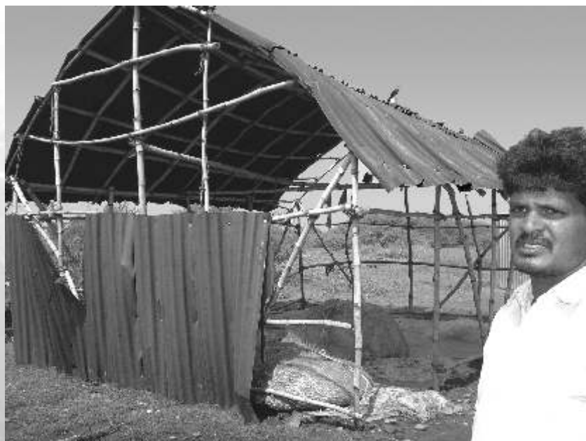
The community center shown above is in a dilapidated state. The tar sheet walls are missing and the frames are tearing apart. Children are likely to get hurt.
