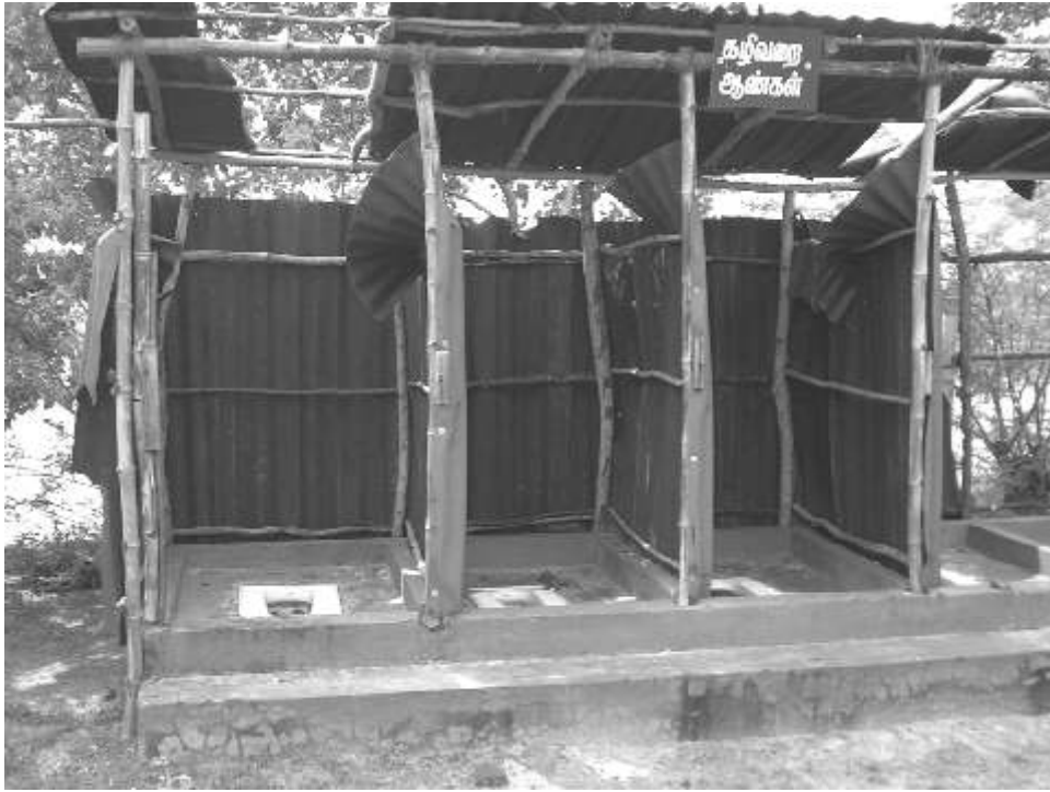
Walls and doors of toilets and bathrooms should be sturdy and must have facility to be locked when in use. Heavy winds can easily blow away the walls and in some cases, doors are missing altogether.
