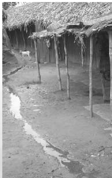
No gutters have been created on the street shown below, and hence rainwater remains stagnant. This not only causes inconvenience in moving from place to place, but there is a large risk of water flowing into the shelters.
