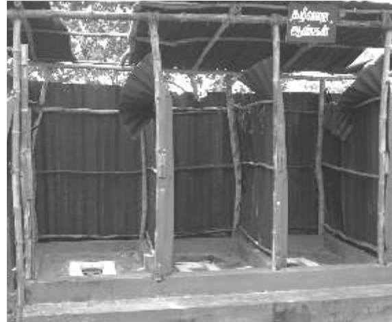
Toilets remain unused because water is not available on a regular basis
