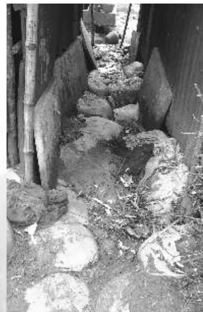
To avoid flooding in between houses, sand bags have been rested against the walls of the shelters. Raising the level of the house with a plinth or creation of drains can reduce the risk of flooding.
